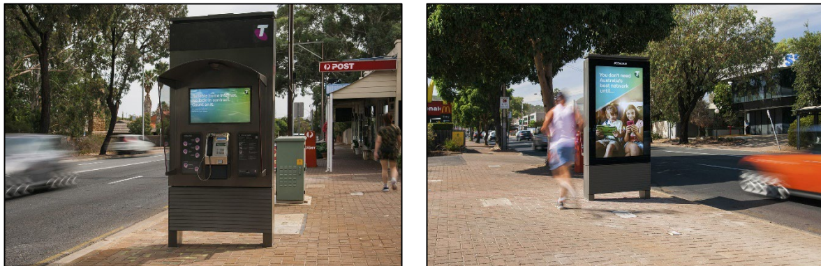
Example Cabinet Installation (Front and Back) [Source: Telstra]
