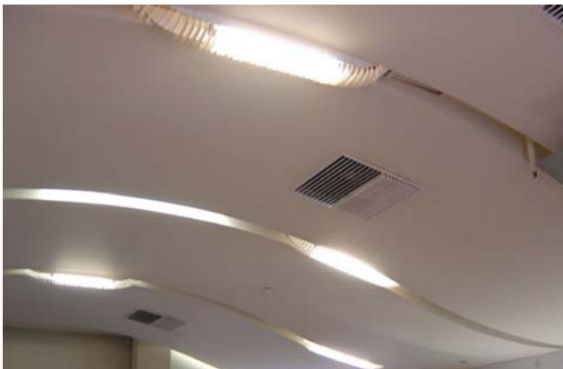
Figure 5: Light fitting mounted on ceiling.
