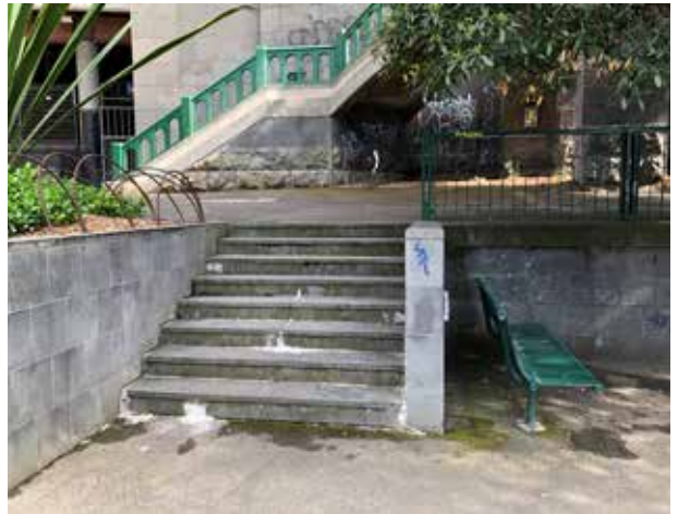
↓ ... poor pedestrian connectivity from street level to the river and lack of universal access ...
