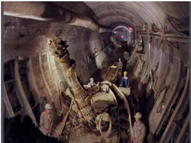
Following the 1969 Melbourne Transportation Plan, the City Loop was completed in 1978. This added an additional rail viaduct along the north bank. [John Holland Constructions, "The Loop" by Wolfgang Sievers, 1977. State Library of Victoria, Accession no: H2004.49/72]
