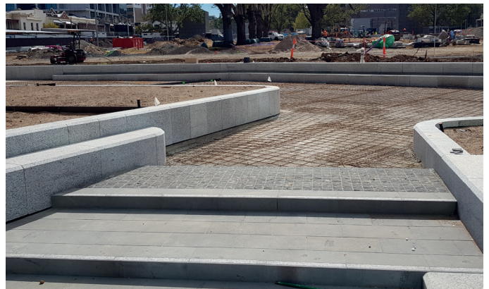
Installation of bluestone and granite terracing is now complete, and final preparations for the concrete pavement are underway
