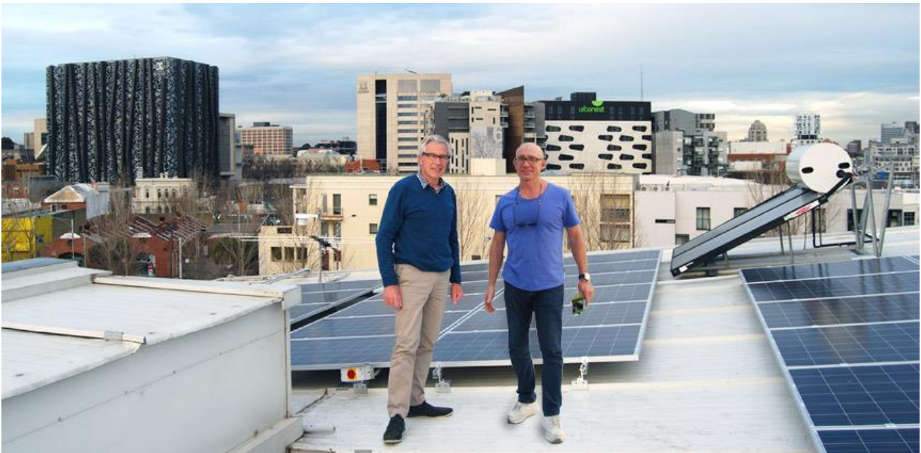
Two of FMSA’s directors, Peter Sandlow and Greg Anson, inspect the new 30kW solar installation system.
