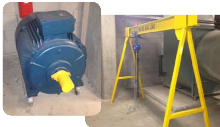
Spare equipment can be stored in convenient locations to minimise downtime, such as this condenser water pump motor and associated lifting equipment. (images courtesy of FMV)
