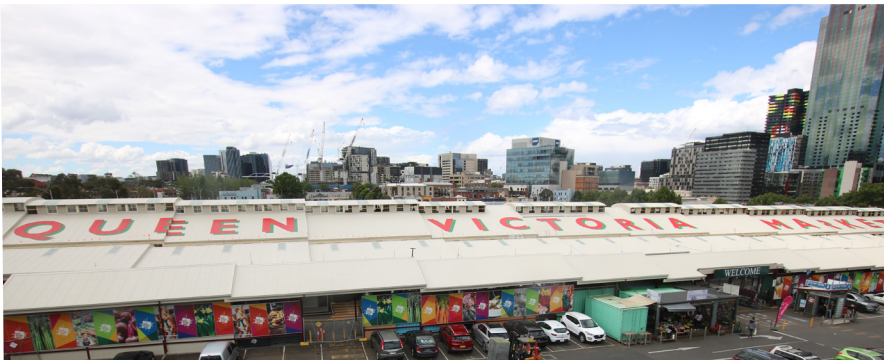
Photo: The new insulated roof on Sheds J to M and repainted signage.
