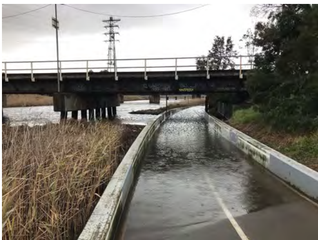
Image 28: Flooding along Moonee Ponds Creek impacting the Capital City Trail during a high rainfall event.
