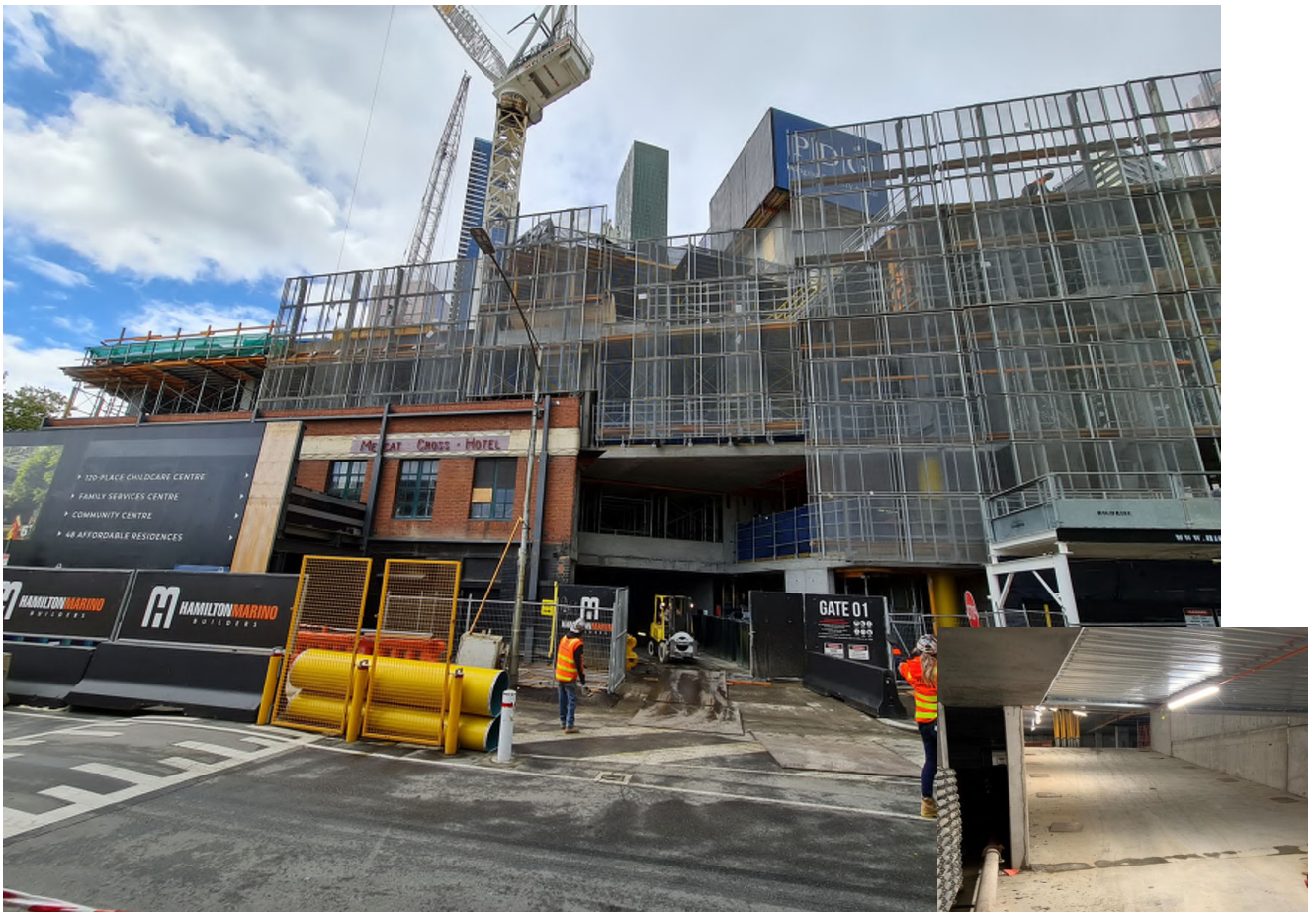
Figure 2 – Street view from Queen Street to the Munro site, showing the entrance to the QVM customer car park. Inset - Ramp between levels of QVM customer car park.
