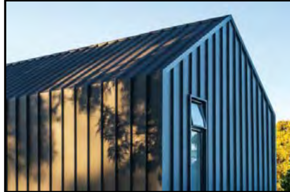
Metal with Expressed Ribs. Darker monument colour used for cladding. Lighter shale grey colour used for roofing for superior solar performance.
