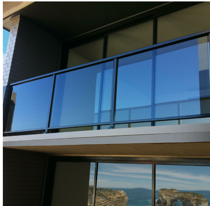
GLASS BALUSTRADING THROUGHOUT DEVELOPMENT, ALUMINIUM FRAMED, FLOOR TO CEILING GLAZING OPTIMIZED FOR THE BEST ESD RESULT. WINDOWS OPTIMISED TO ALLOW BEST LIGHT INTO SPACES WITHOUT ALLOWING EXCESSIVE HEAT LOSS.
