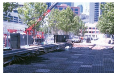
Stormwater harvesting at Queen Victoria Market
