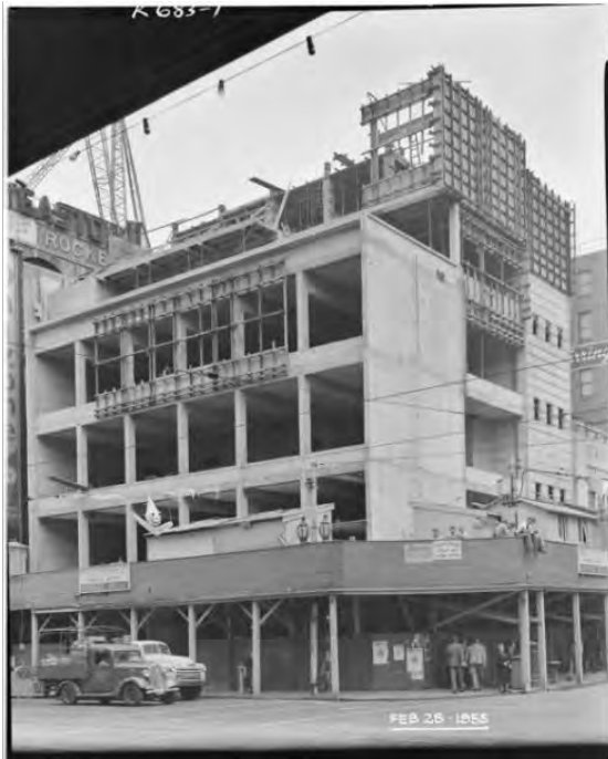
Figure 4. The hotel under construction in February 1955 (SLV, Lyle Fowler, photographer, Image H92.20/5269).
