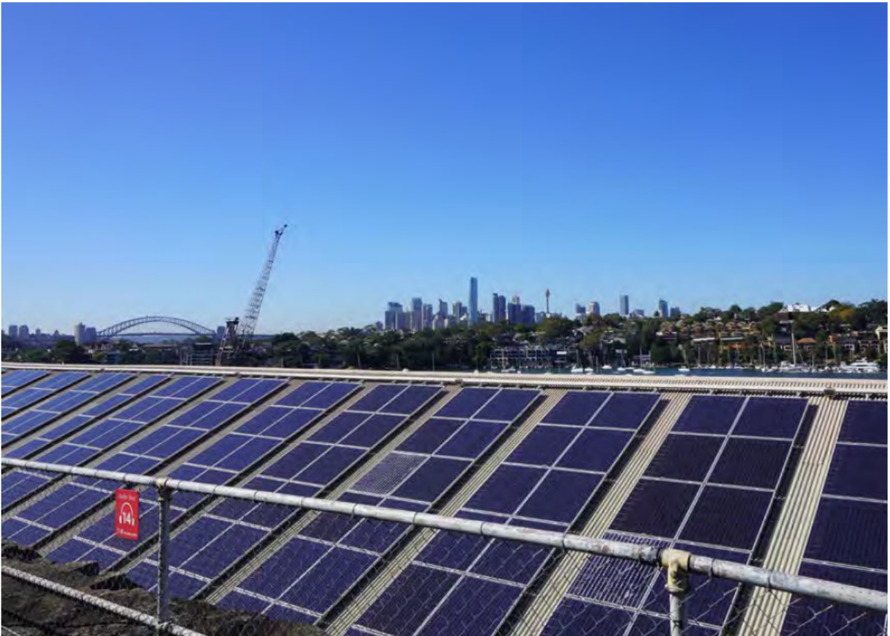
Figure 15: Solar panels on Turbine Hall, Cockatoo Island, New South Wales.
