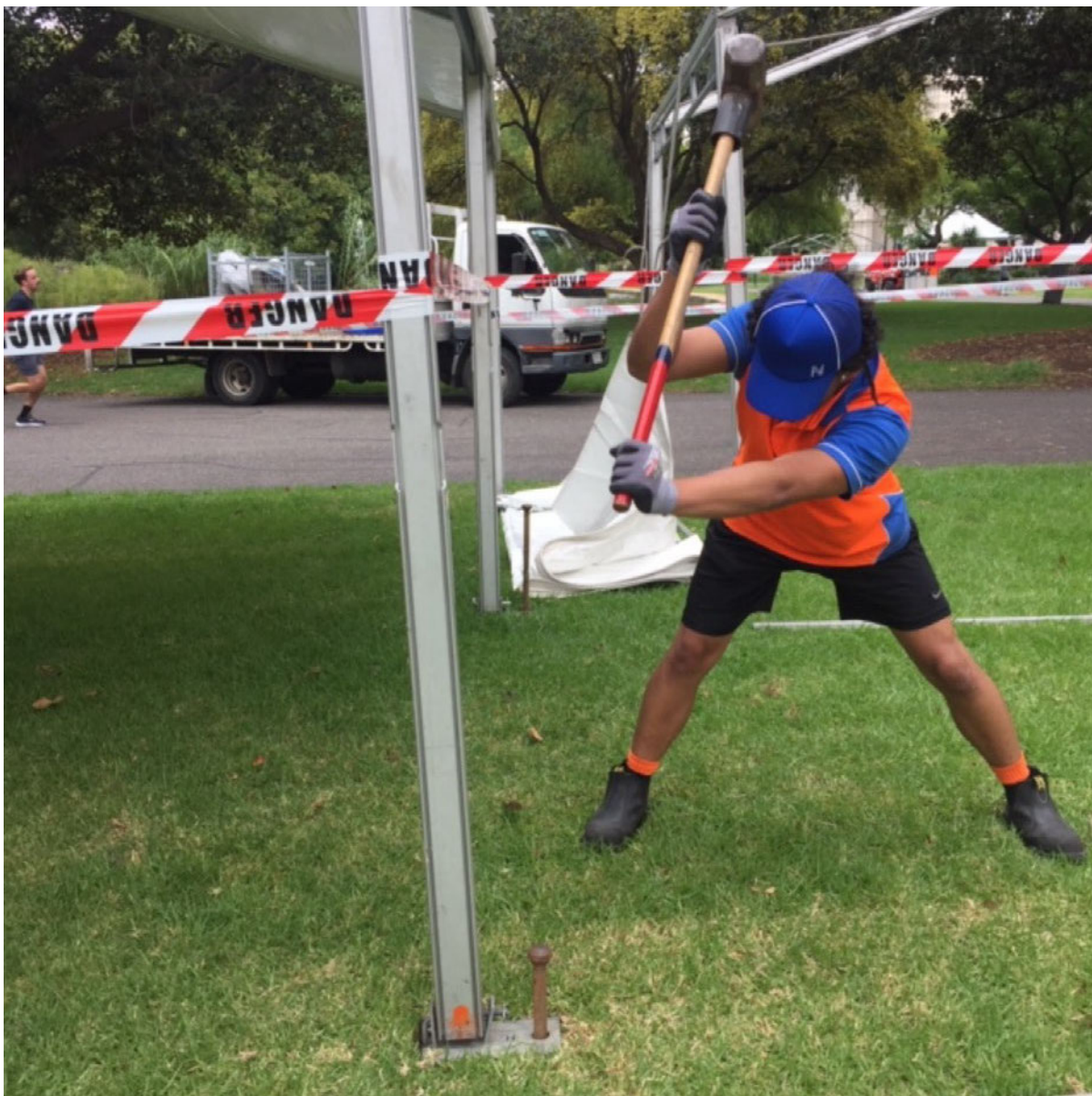
Hammering in spikes directly under a tree. These spikes can pierce roots.
